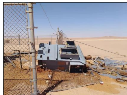
Damages at the station
