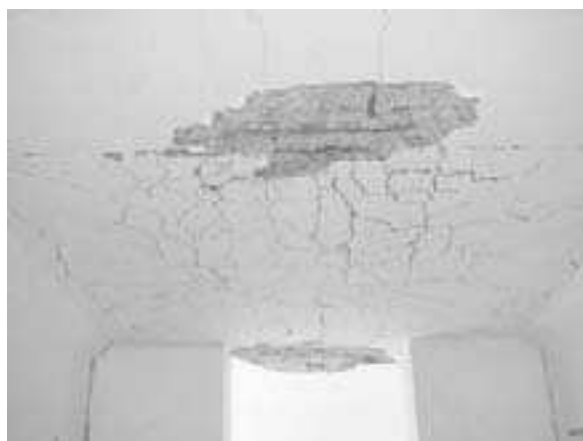
(b) Post-test showing roof inside with minor spall damage.
