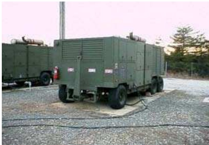
Figure 11-2. Prime Power generator
